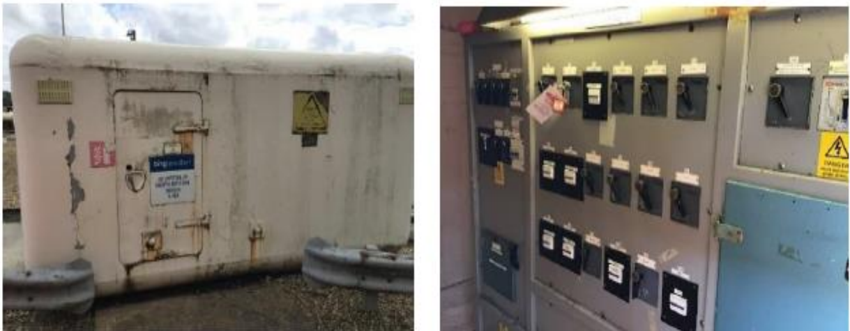
Figure 6: Kiosk F (left) and panel (right)
