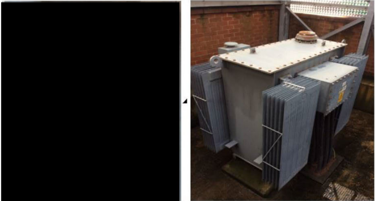
Figure 2: LV Transformers Technical Specifications (left) and Transformer picture (right)
