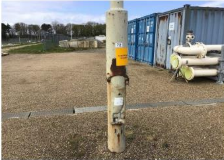
Figure 7: Typical lighting column
